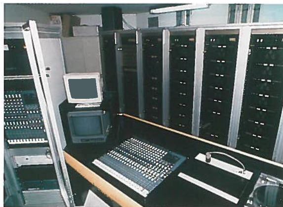
Soundtracs FMP installed in the Great Mosque in Casablanca.
